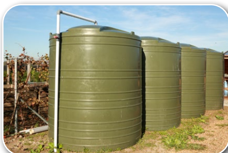
Rainwater harvesting tanks
